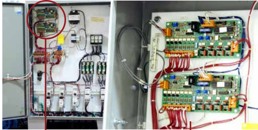
Zone Board location inside electrical cabinet.
