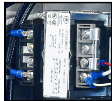
Control circuit transformer fuse
