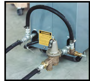
Typical pressure reducing valve installation (shown on S-925 model).
