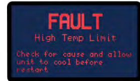
High Temp Limit Fault Screen.
