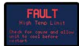
High Temp Limit Fault Screen.
